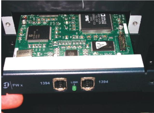
Installing the FWx card in the FOH Rack
